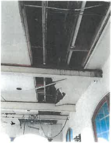
STRUCTURAL ROT AT DECK
